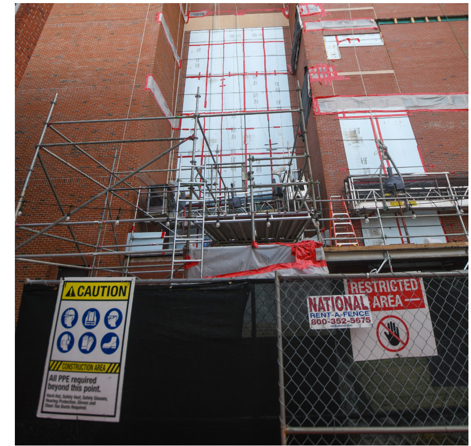
The side of D.H. Hill Library is being worked on on Feb. 17. The Brickyard has seen major demolition in preparation for the construction of the new Integrative Sciences Building.
