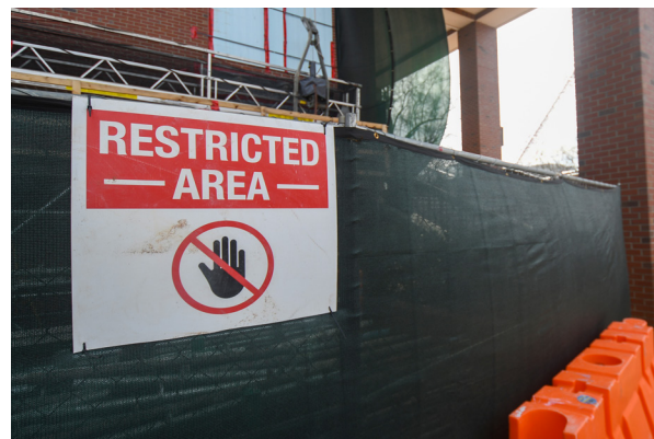
A sign restricts pedestrians from entering a construction zone outside of D.H. Hill Library on Feb. 17. According to the library website, the building received major renovations that were completed in 2020.
